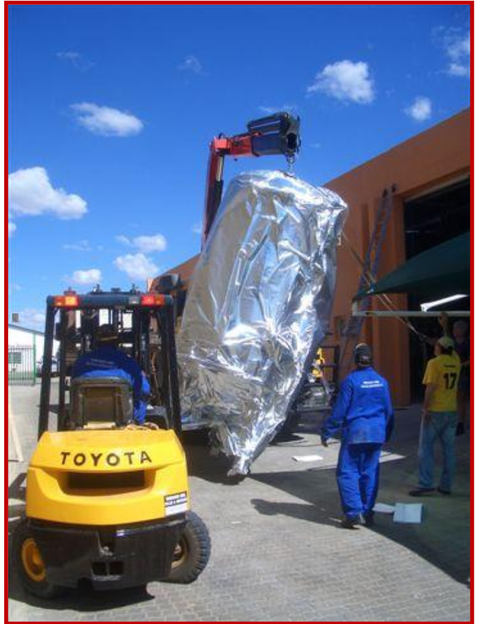
Tank being loaded in Germany (March 09) and unloading in sunny Namibia, 26 April 2009
